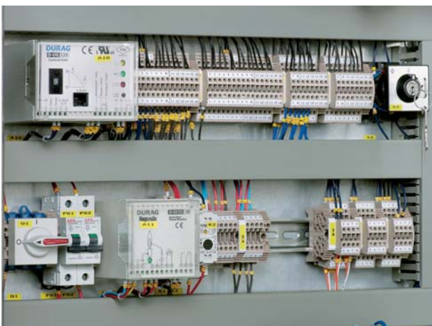
BMS safety devices.
