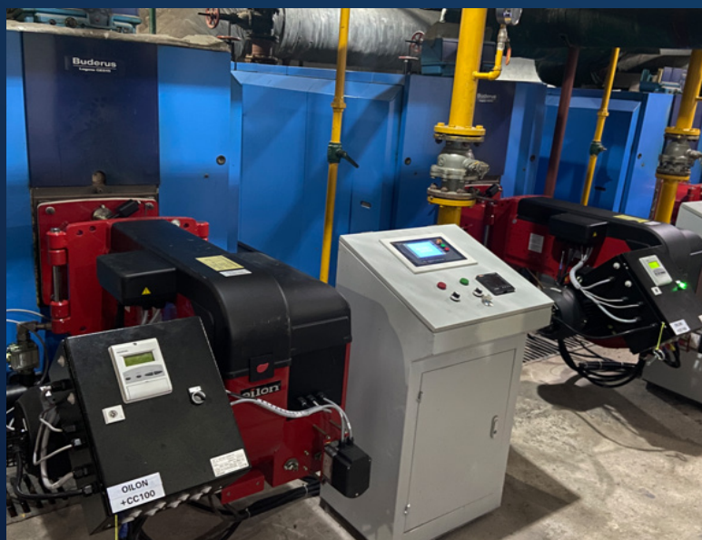
3 x GP-250 M LN30, burner capacity 1 400 kW
