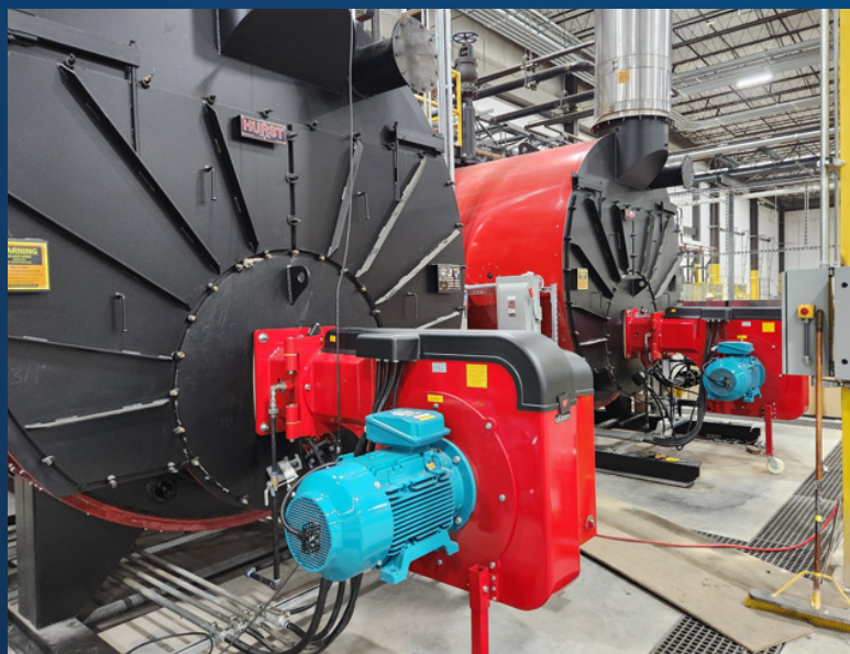
2 x GP-600 M-II LN30, burner capacity 5 400 kW
